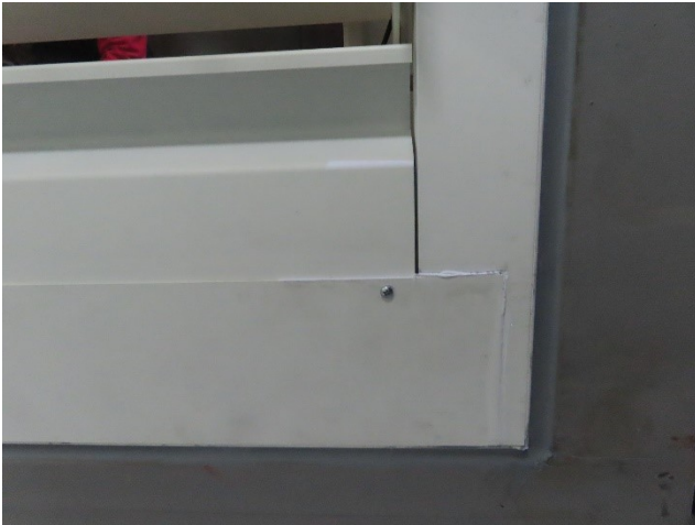
Picture 3 Corner of test specimen
