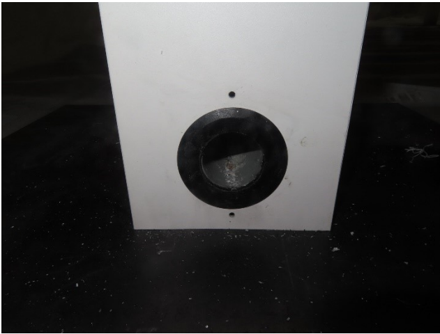
Picture 7 Drainage system
